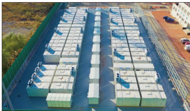
Figure 17. General view of the energy storage system based on vanadium flow battery (5 MW/10 MW h) in Shenyang, China. (Rongke Power; https://rpkstorage.com/projects/ accessed on April 1, 2026).
